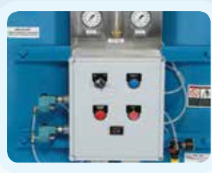
NEMA 4X Control Box
